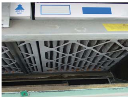
PHOTO A. Filter gap.
