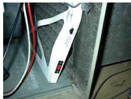
PHOTO B. Improperly sized filter.
